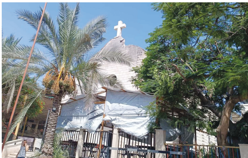
Damage can be seen next to the cross on the roof of the Holy Family Church in Gaza after it was hit in an attack July 17, 2025. (CNS photo/courtesy Aid to the Church in Need, UK)
